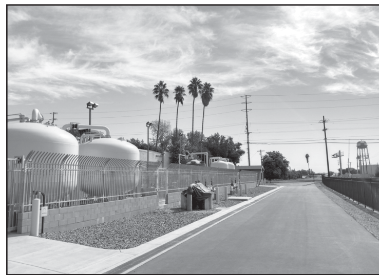
The Arden Ground Water Treatment Plant has a capacity to treat 750 gallons per minute. The Plant treats groundwater by filtering it through two stages of carbon.
