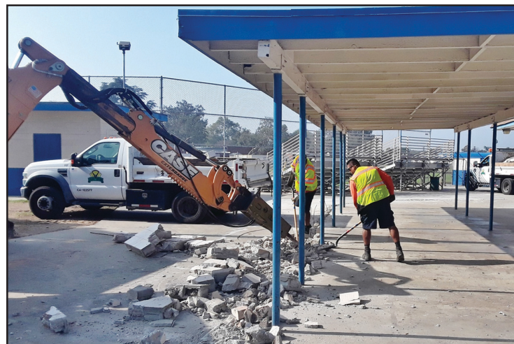
Destruction of certain areas at Del Norte Park took place because of the transients and homeless that took over parts of the park.
