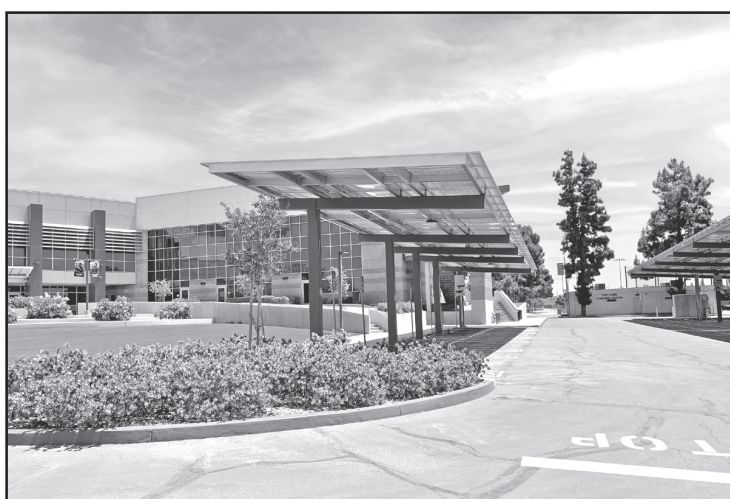
Solar panels cover the Citrus College E2 and portions of the S2 (south of the Student Services Building) parking lots. Solar power provides a more efficient way for the college to meet its energy needs. (Photo courtesy Citrus College)
