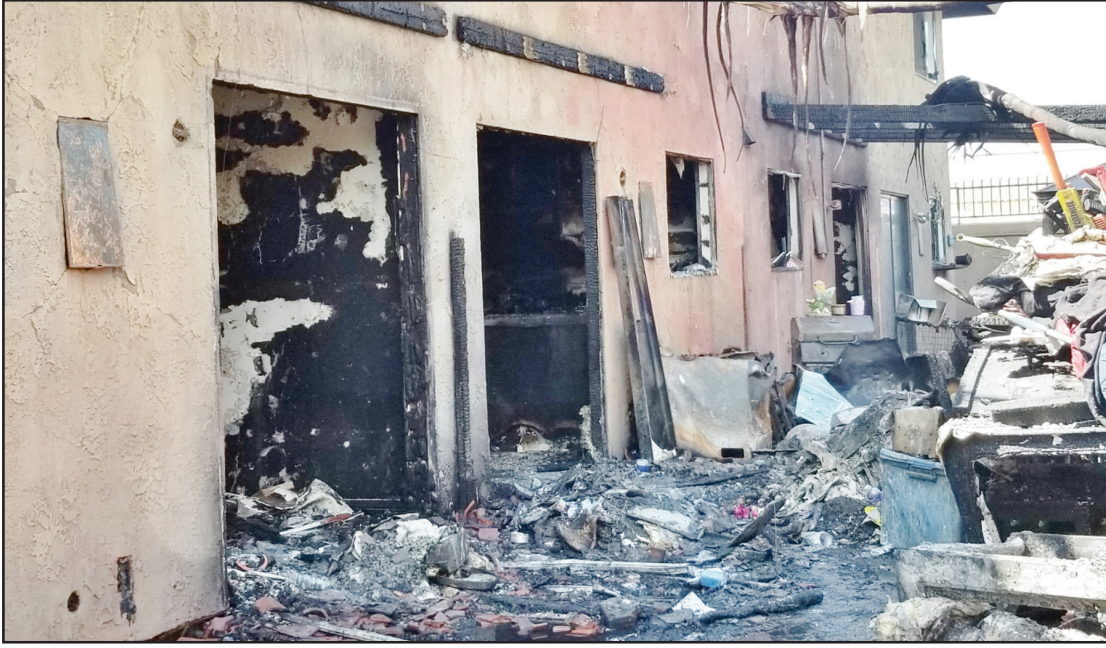
All units lost as the fire burned from the garages (right out of picture) to this void area which had patio covers.
