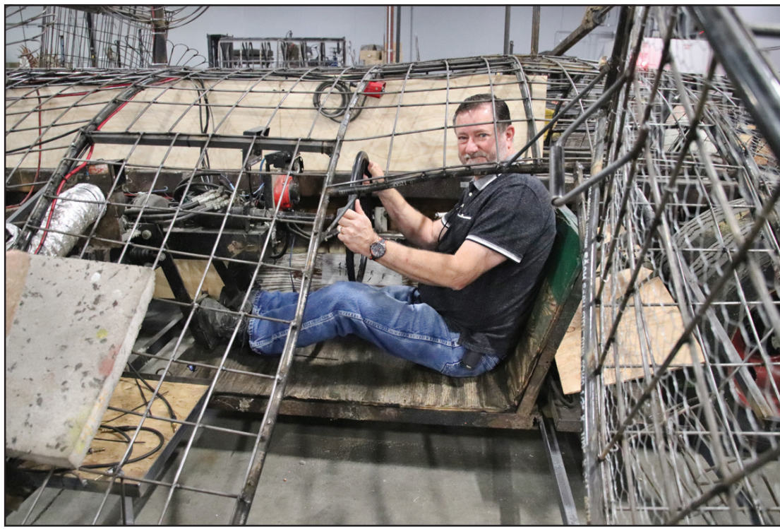
Bud checks out his driving space during float construction. (Photo by Jean Palmer)
