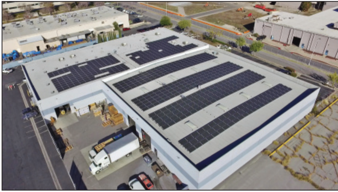
Mortech Manufacturing facility in Azusa with solar panels installed by SunGreen Systems.
