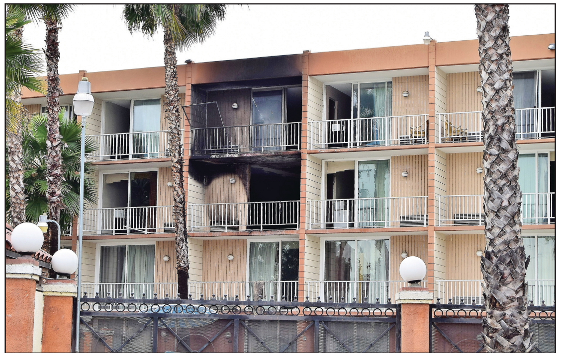
Damage shown as the result of the fire at the Regency Motel in Baldwin Park. Building has been "Red Tagged" until further notice.
