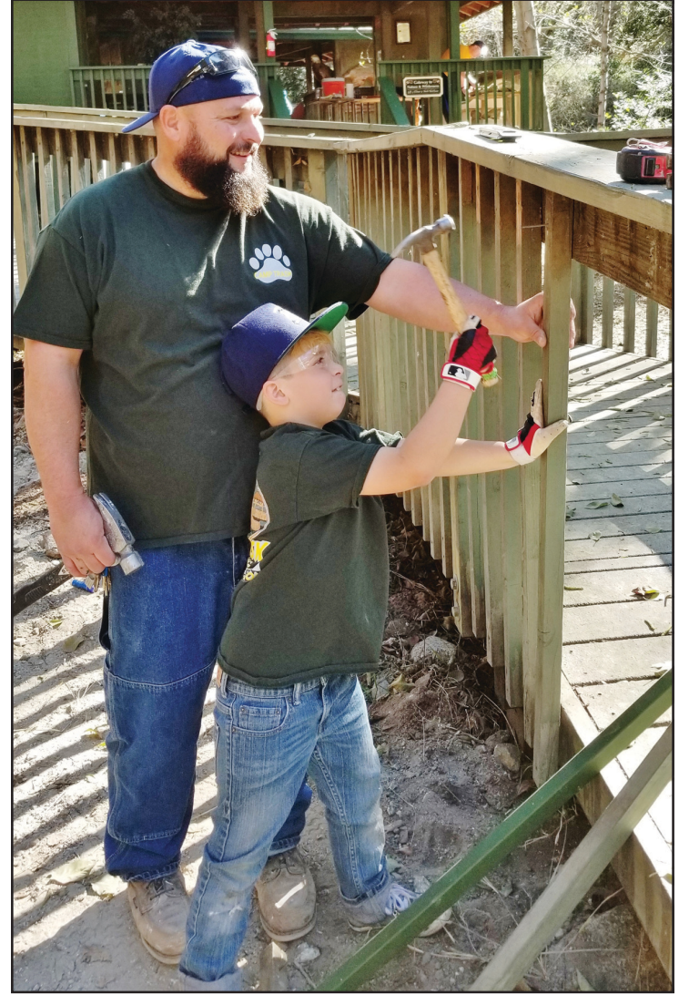
Pack 66 Tiger Den Leader David Gomez with Tiger son Aiden repairing the handicap ramp
