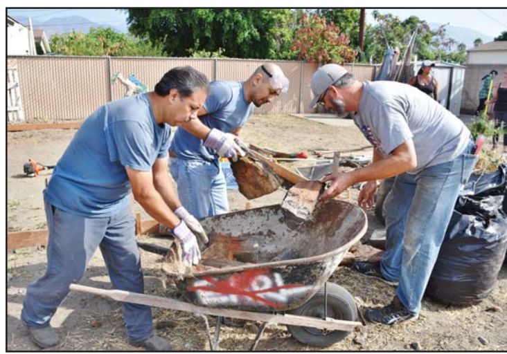
In order to expedite the removal of debris from the back yard to a dumpster located in the street, volunteers of the Neighbors Helping Neighbors program make use of a wheelbarrow to take the debris to the dumpster.
