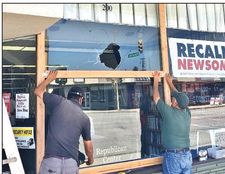
Workers are seen in the process of covering the broken window with plywood. Replacing the glass will not be accomplished until a sufficiently large pane of glass can be located.
