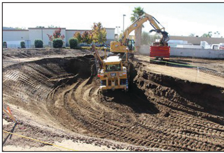
Crews excavating for the pedestrian undercrossing that will provide riders access to the Glendora station platform from Glendora Ave.
