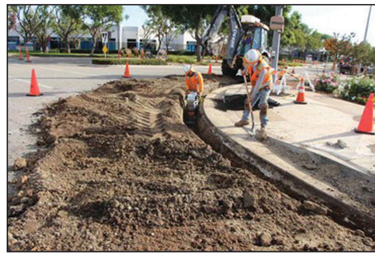
Crews installing underground conduit to provide power to new traffic signals at Wheeler Ave./Arrow Hwy.
