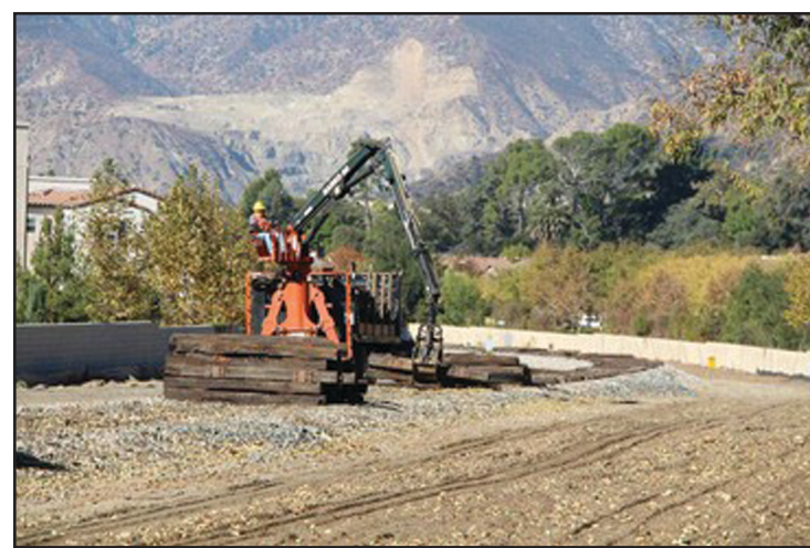
Crews using specialized equipment to remove freight track piece by piece in Glendora
